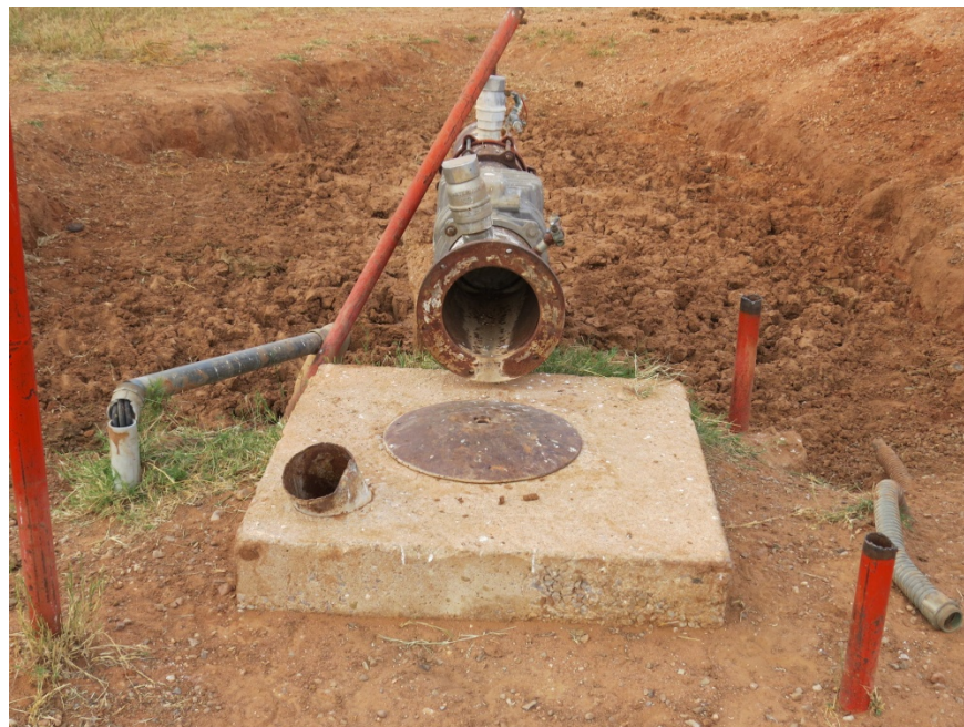
Photograph #8. Wellhead and vent pipe in concrete pad surrounding wellhead for the agricultural well in the northeast quarter section, looking west. A metal plate has been placed over the wellhead. Vent pipe is uncovered but is filled with soil
