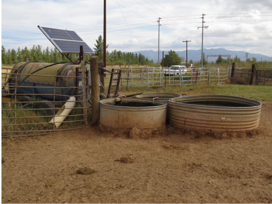
Photograph #3. Three livestock tanks are adjacent to the south of the first wellhead. Solar panel provides power for water pump. View is to the east northeast.
