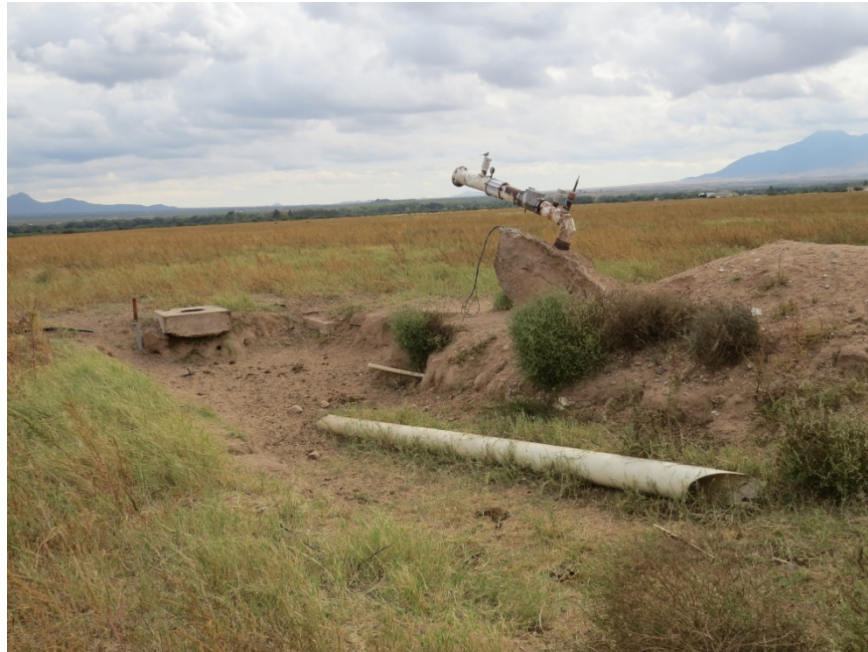
Photograph #11. The photograph of the excavated distribution system for the agricultural well in the southeast quarter section is taken looking to the southeast. Eight inch PVC piping was used to convey water to center pivots.
