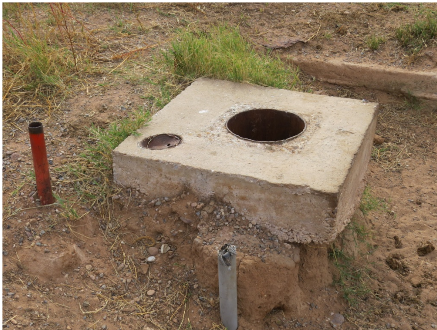
Photograph #12. This photograph of the wellhead for the agricultural well in the southeast quarter of the section, looking to the south southeast. Wellhead is open, with vent pipe covered but in poor condition. Electrical cable pipe is in the foreground.
