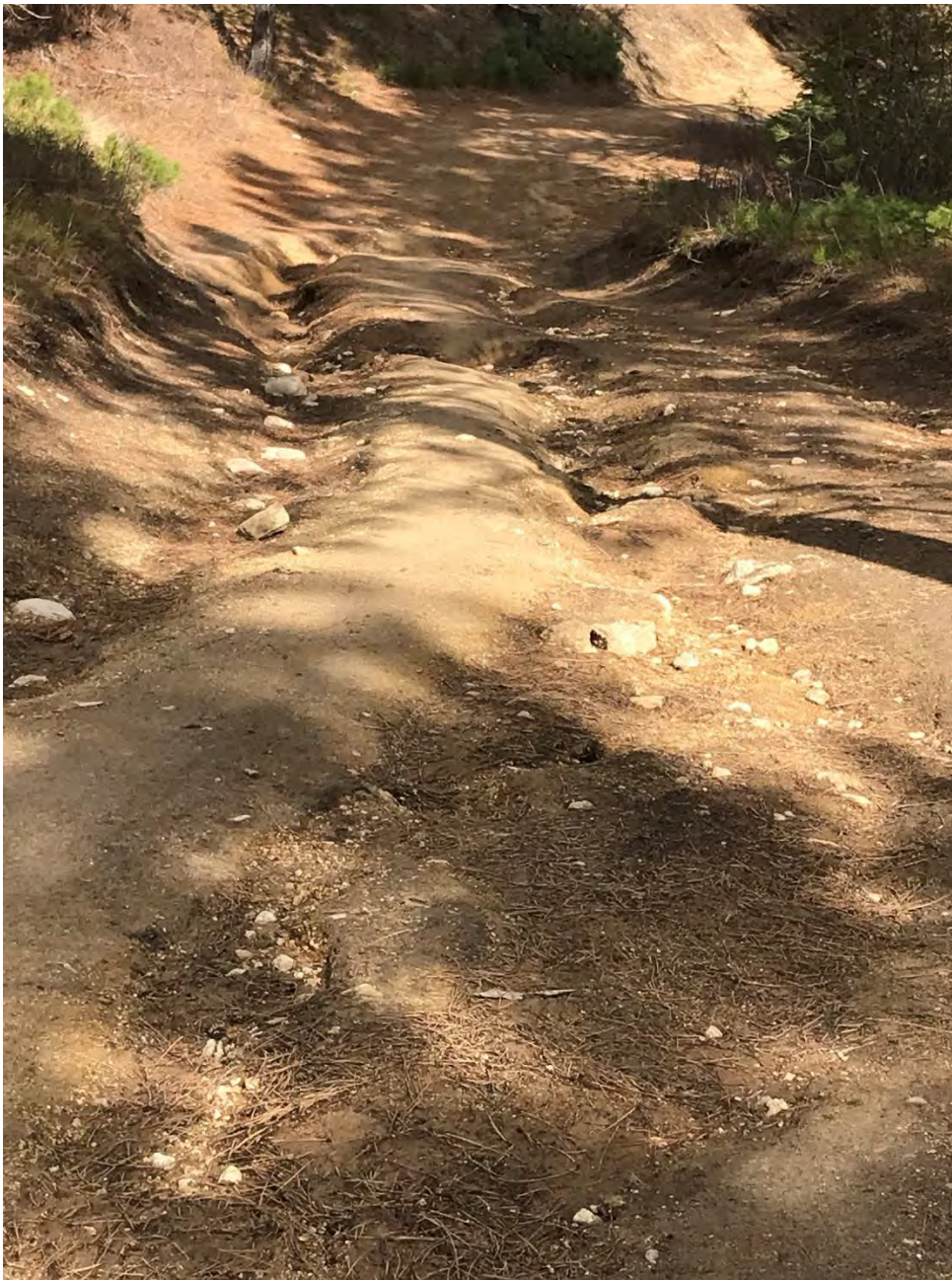
3-22-2024 view of FR 74964, the access road to trail 511 and the Westside project road to unit 2c. No maintenance has been done since the Westside commercial harvest concluded, and it is now impassible to passenger cars.
