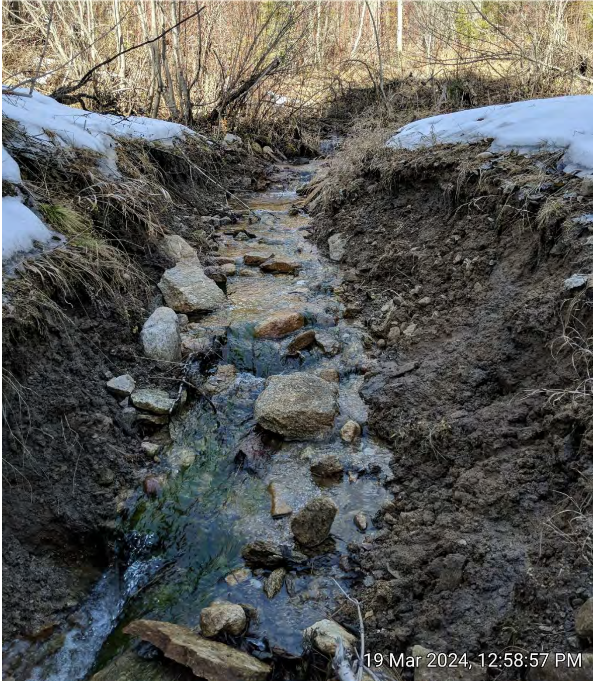
Culvert removal along reclaimed FR 5620 showing the eroding vertical banks that were left. This is the main branch of Moose Creek, a perennial tributary of Lost Horse Creek.
