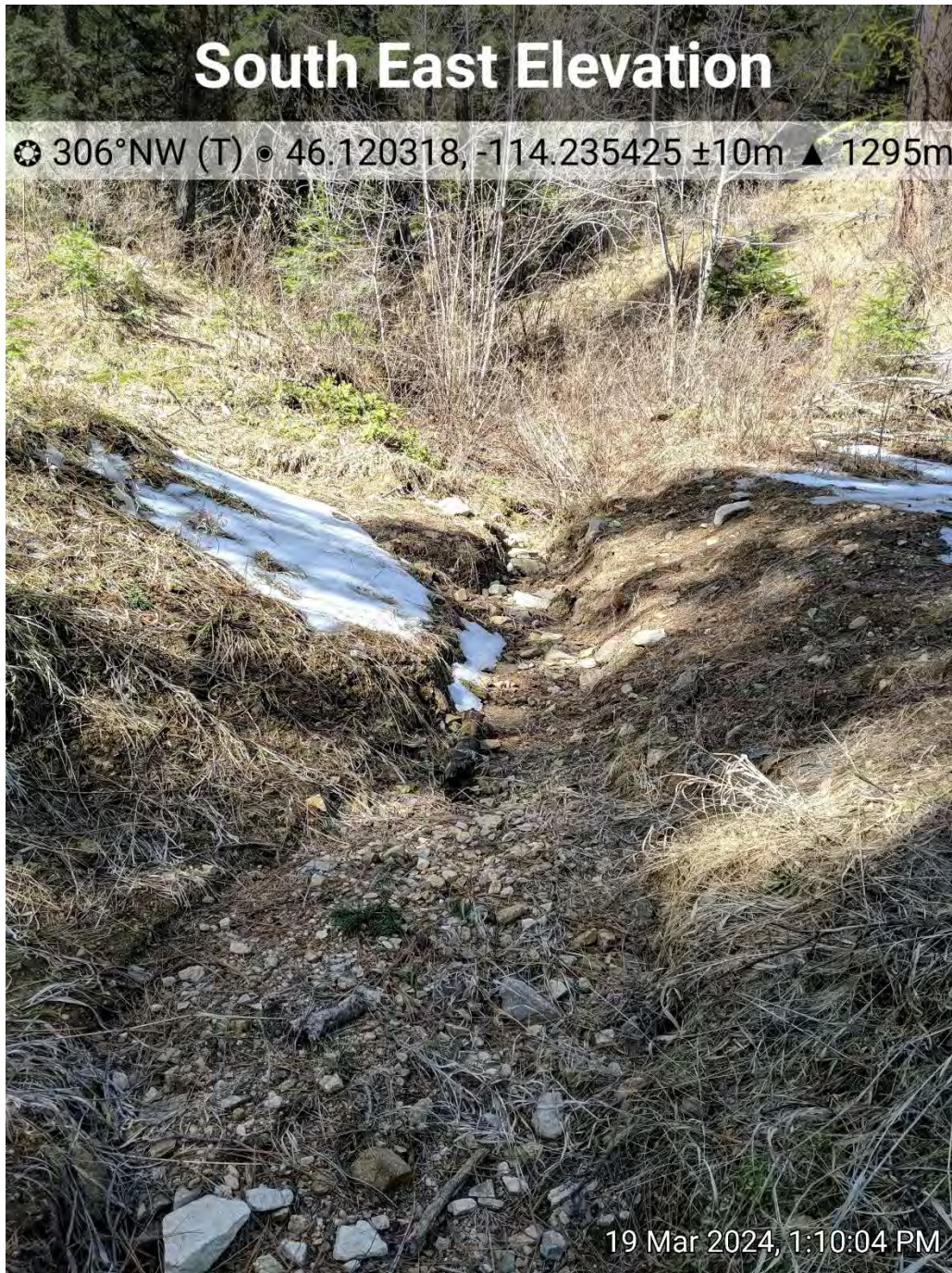
Another culvert removal where FR5620 crossed an intermittent stream where no recontouring or reseeding was done.
